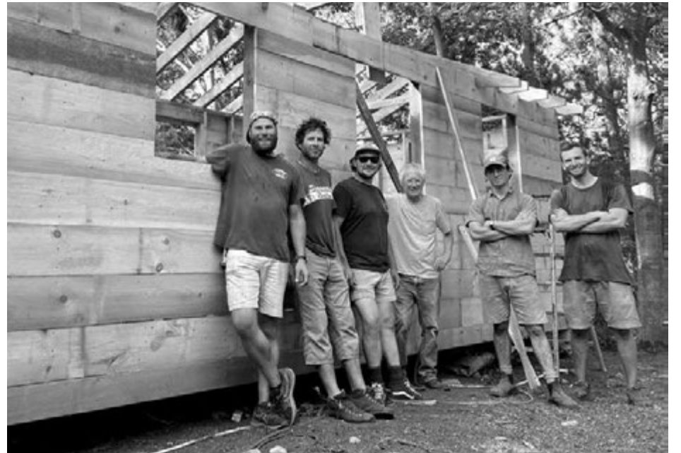
The volunteer crew during construction, September 2022. (Left to right) Peter, Jim, and Tom Nagler, Tom Yoder, Miles Frank, and Rip Swan.
