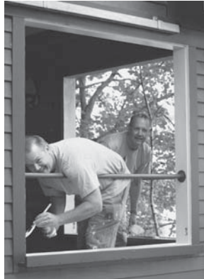
Pope and Peter judgmentally touch up paint work done by other volunteers.
