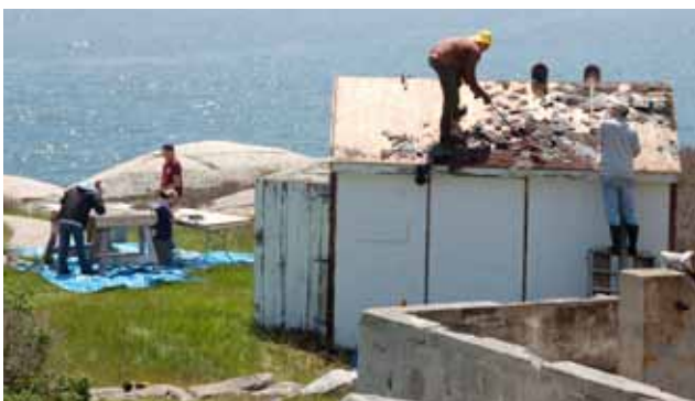
The beginning of the tractor shed to staff quarters project at Whitehead Light Station
