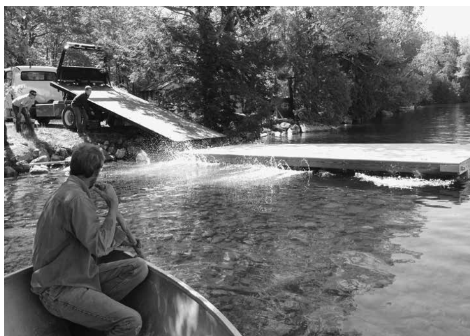
Shed City’s truck drops the new floating dock into Great Pond in the early spring.
