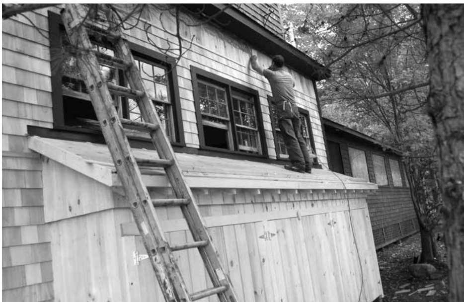
Carpenter Dan Trembly at work atop the new trash shed in front of the kitchen
