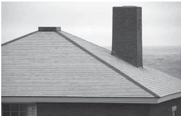
Repaired chimney and new roof with copper caps on ridge and peak
