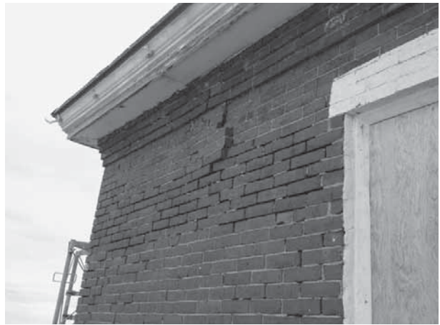
Crumbling bricks and deteriorating soffit on the east wall of the Whistle House
