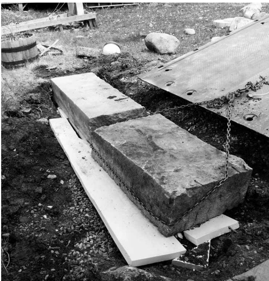
Granite blocks to anchor the platform to which the ramp is attached
