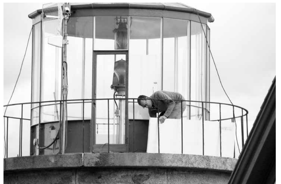
Matt Wall at work on the storm door for the lighthouse lantern deck
