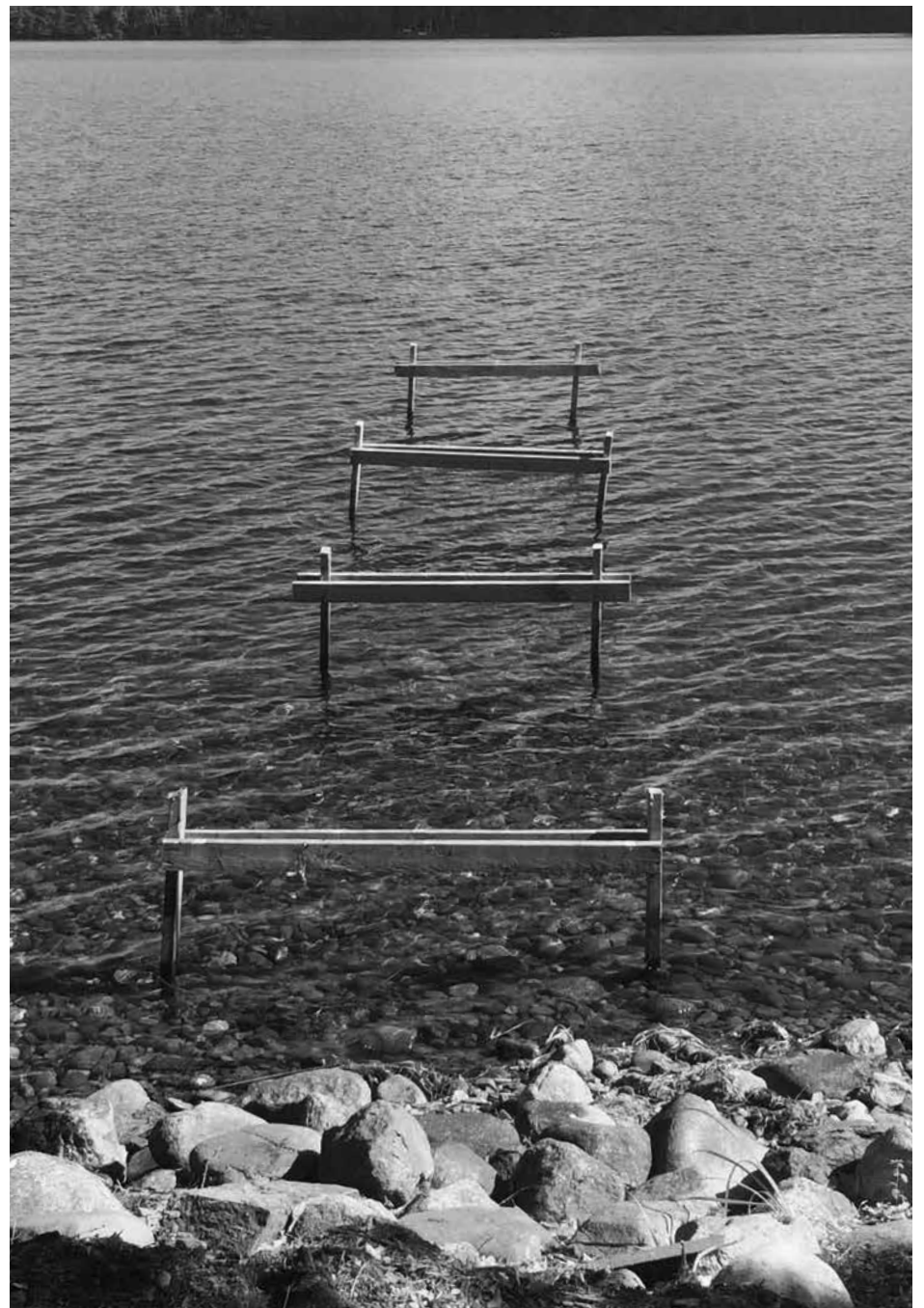
Out with the old: the last of the old Kitchen Dock ready to be removed
