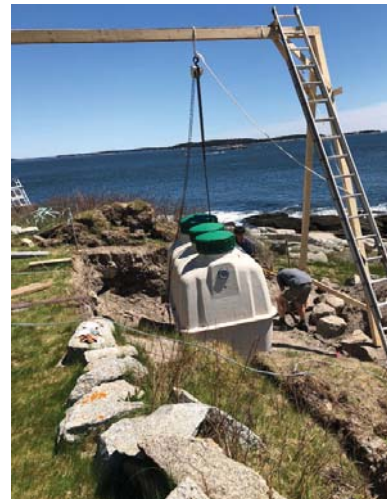
The new sewage treatment tank is lowered into the ground in front of the Whitehead Lighthouse
