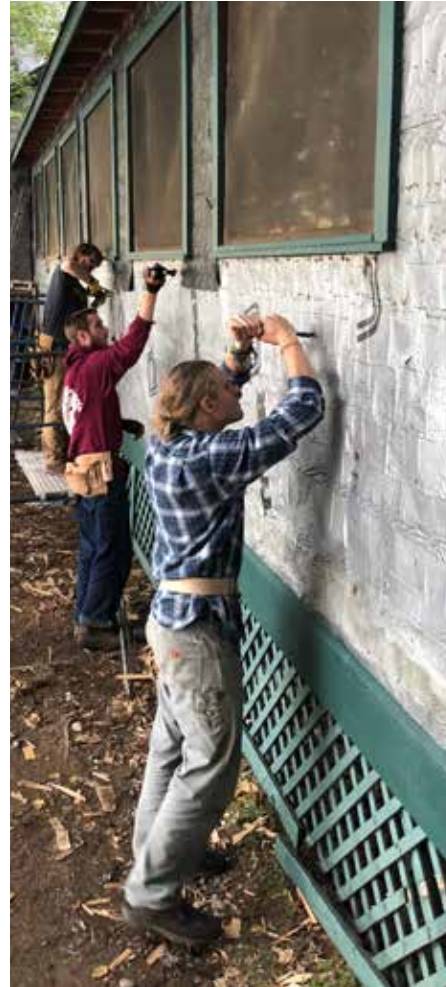
Sam Bristol, Cole Gibson, and Satchel Toole preparing the Dining Hall for reshingling
