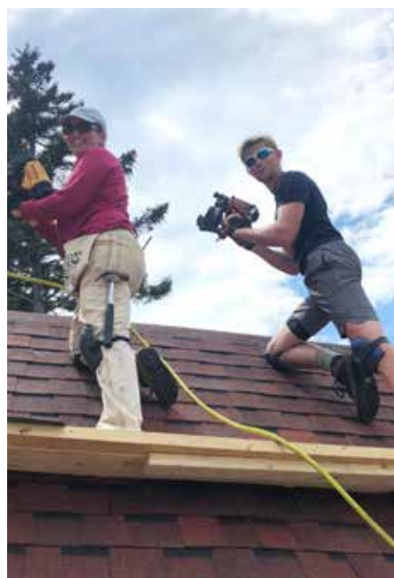
WLS Director Gigi Lirot and intern Thomas Clauson celebrate finishing the boathouse roof.
