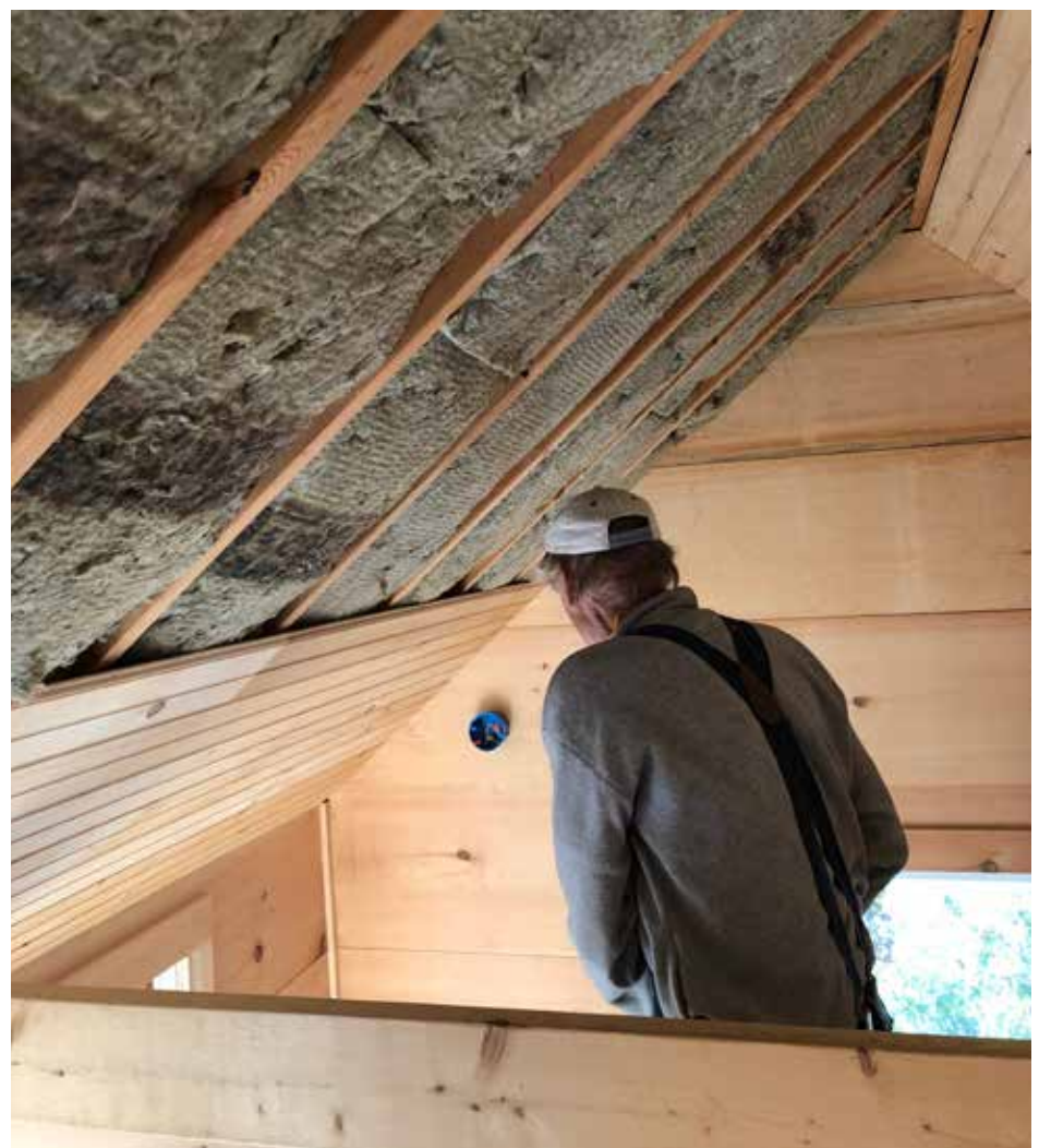
David Pope at work on the interior of Hilltop House at Whitehead Light Station
