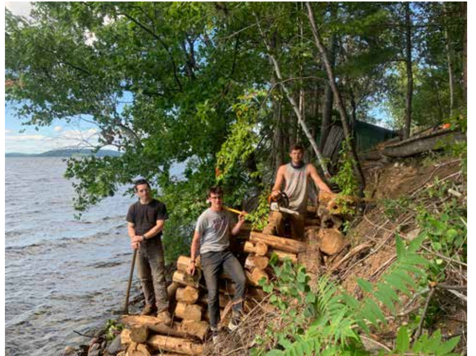
Miles, Bobby, and Justin with new cribbing to prevent further erosion on the West Range
