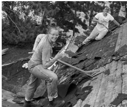
Fall Crew members Hannah Gordon and Kaja Surborg prepare the Boathouse for its new roof.
